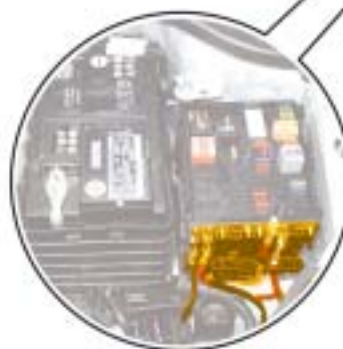
Strip fuses in the fuse and relay box
