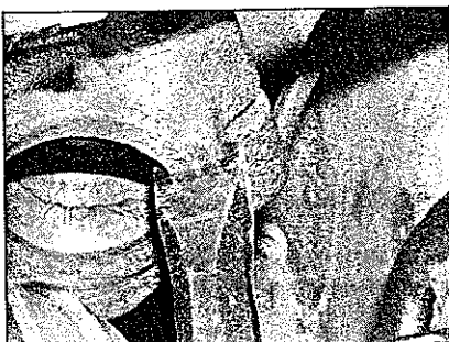
2.10b Using a cold chisel to open up the wheel bearing housing and release the suspension strut
